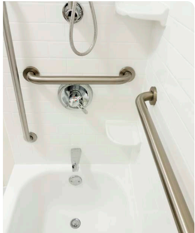
For your safety, you may need to have handrails installed in your bathroom.
